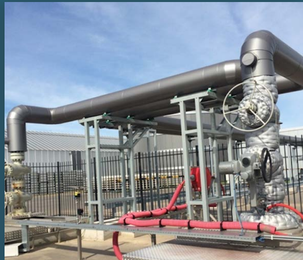
Bovenstation geothermie put 10-30MW
